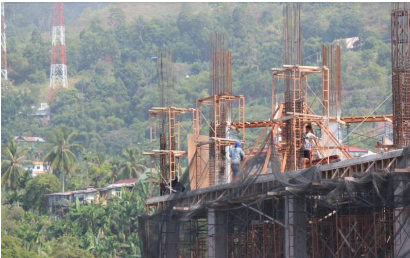
Construction underway in Jayapura, the capital of Indonesia's Papua province, in 2015. (Johnny Blades)
